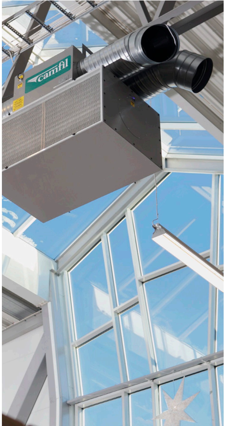
A ceiling-mounted air purifier efficiently purifies the air of nanoparticles as well as of large visible bits of dust. At the same time, the air is remixed, which provides a higher average temperature at floor level.
