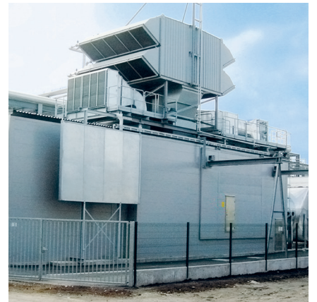
Filter house for enclosure ventilation on a Siemens SGT 800 gas turbine.
