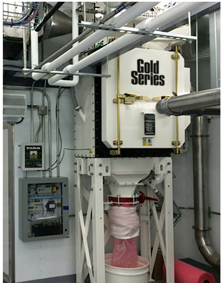
The GSC2 sits in one section of the POD, which is divided up into six sections.
