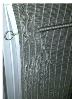
Tri-Dim Damaged Filter
